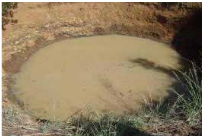
Figure 6: On-farm ponds affected by poor workmanship. Photos: S. Ngigi.
