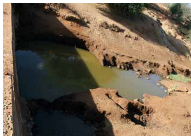
Figure 36: Sand storage dam affected by seepage losses. Photo: J. De Trincheria.
