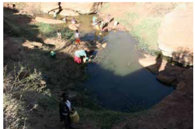
Figure 27: A sand storage dam with severe problems of seepage. Photo: J. de Trinchieria.
