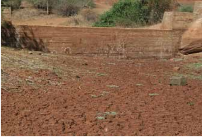
Figure 25: A sand storage dam severely affected by siltation (left) and universal dynamics of fluvial sediment transport (right). Photo: J. de Trinchieria.
