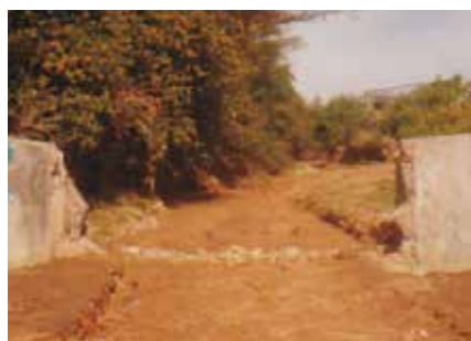
Stage 4: Flood has deposited sand to the new level of the spillway
