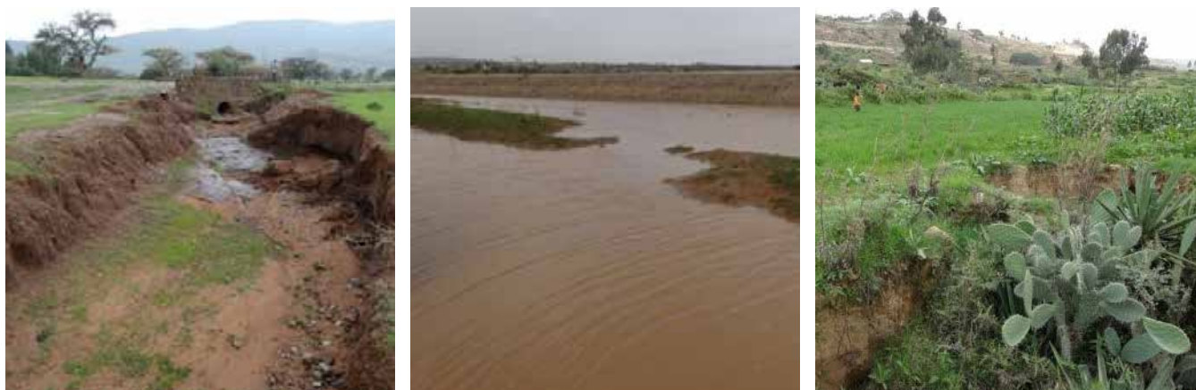
Figure 38: Damage from roads: gulying (left), water logging (middle) and sink holes (right). Photos: MetaMeta.
