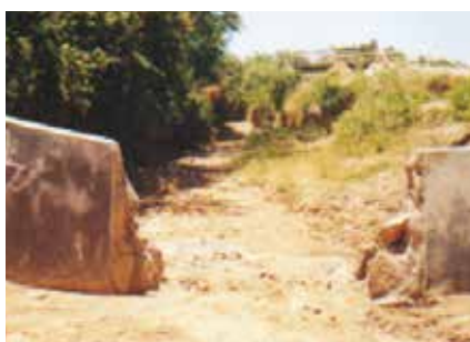
Stage 2: Flood has brought sand to the level of the spillway.
